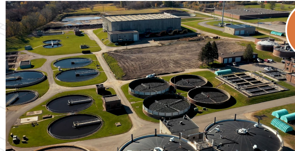
Designing for more flow and industrial loading variations for one of Minnesota's largest phosphorus point-sources.
